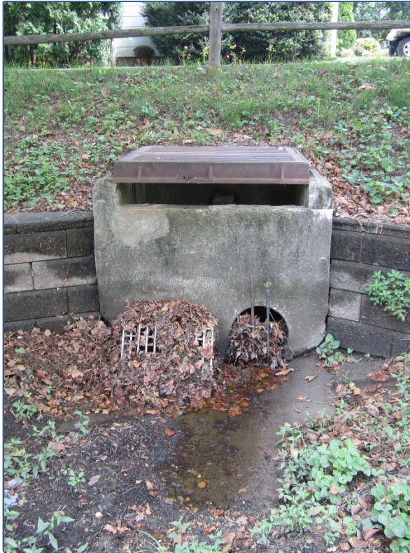
Outlet blockage by debris
