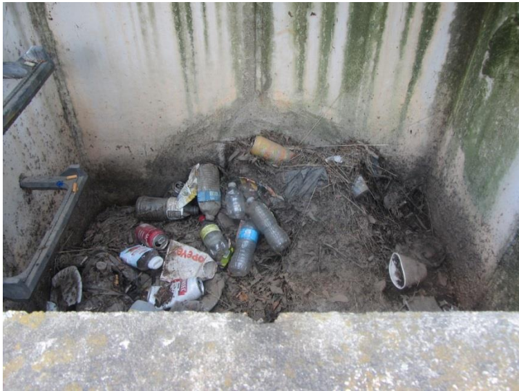
Accumulation of floatables from outfall
