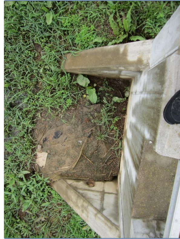
Outlet blockage by sediment
