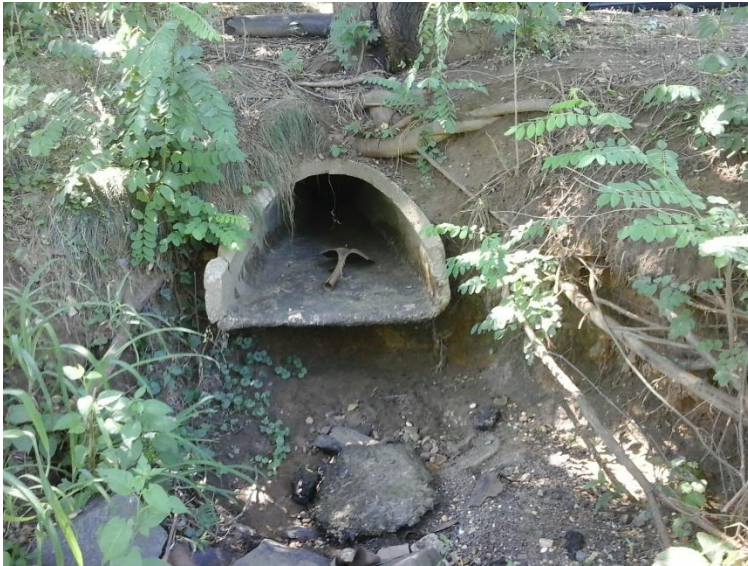
Outfall is causing erosion
